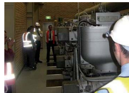
132kV switchgear at Bella Vista
